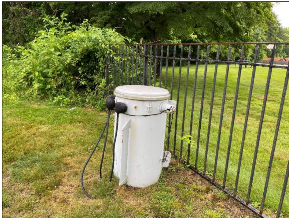
Photo 22: Transformer on the ground next to the fence on the Woods School Property, facing north.
