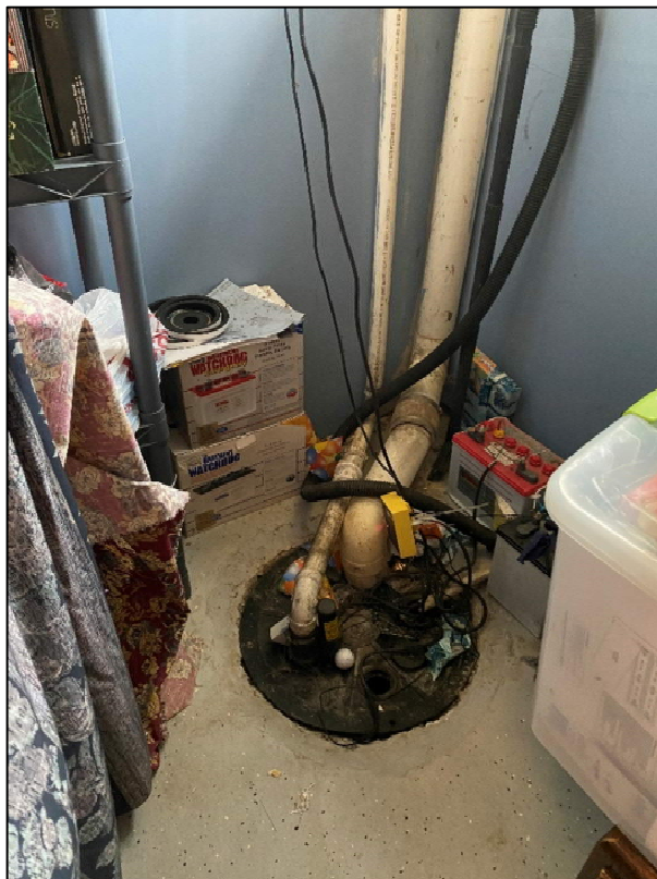
Photo 66: Sump pump located in the basement of the residence.
