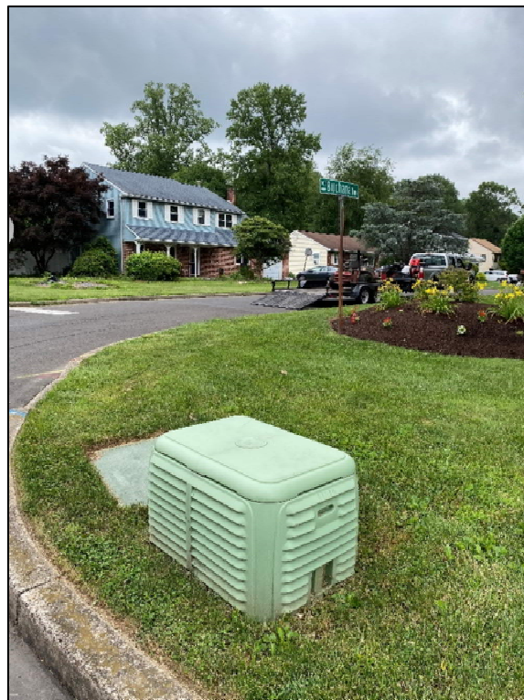
Photo 4: Telecommunications box on the corner of Highland Avenue and Buchanan Drive, facing east.
