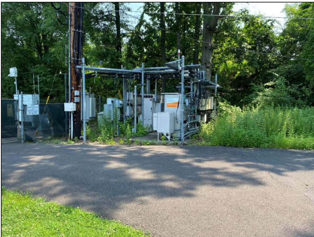
Photo 79: Electric substation at the east end of Central Avenue, facing northeast.
