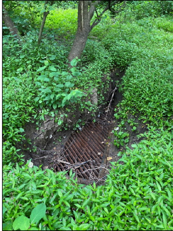
Photo 3: Stormwater grate in the middle of the wooded area along W Highland Avenue between the Delaware Quarries Langhorne Stone property and Park Avenue.
