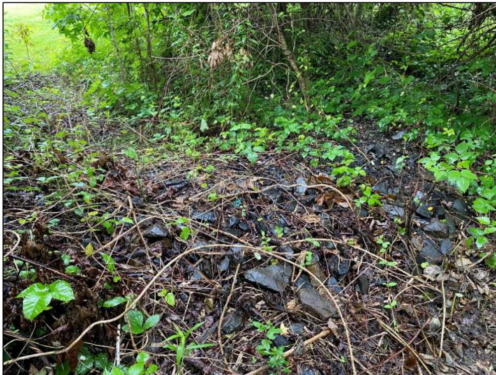
Photo 18: Approximately 12 feet by 3-foot mound of fill material about 2 feet high on the Woods School Property near Pine Street.
