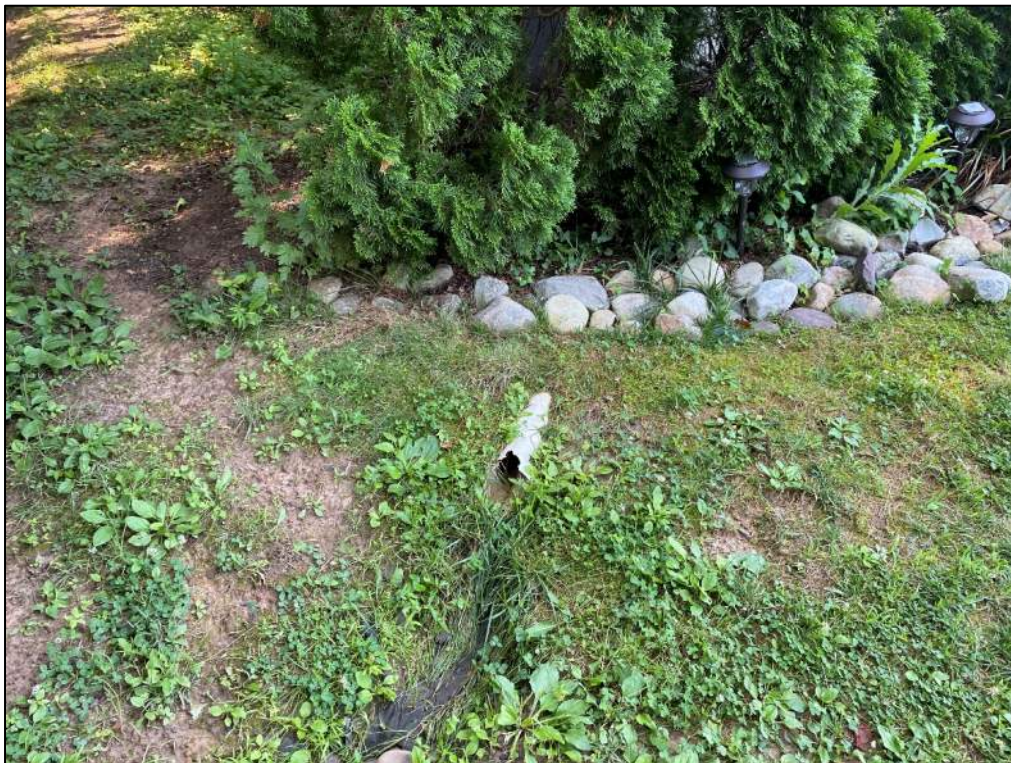
Photo 57: Sump pump drainpipe in front yard of the residence.
