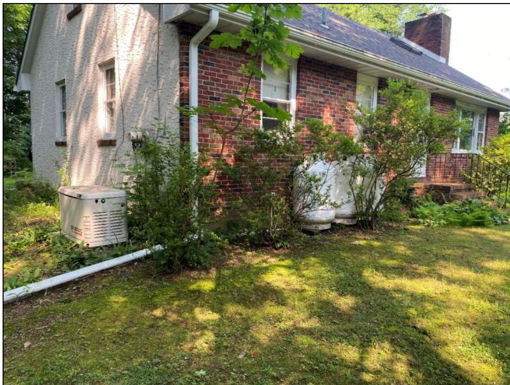
Photo 62: Generac generator on the side of the house and propane tanks in the front of the house, facing west.
