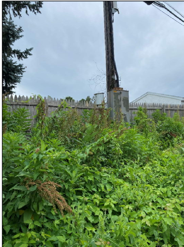
Photo 8: One pole-mounted transformer and a pole-mounted electric box along edge of project area, facing south.
