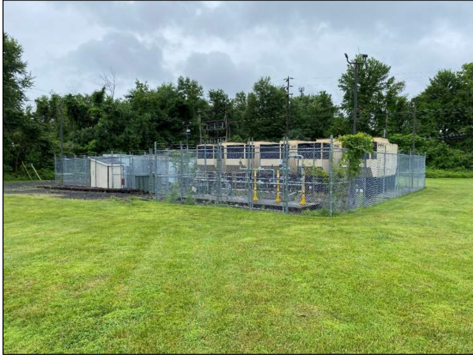
Photo 19: Fenced in electrical substation on Woods School Property, facing southwest.
