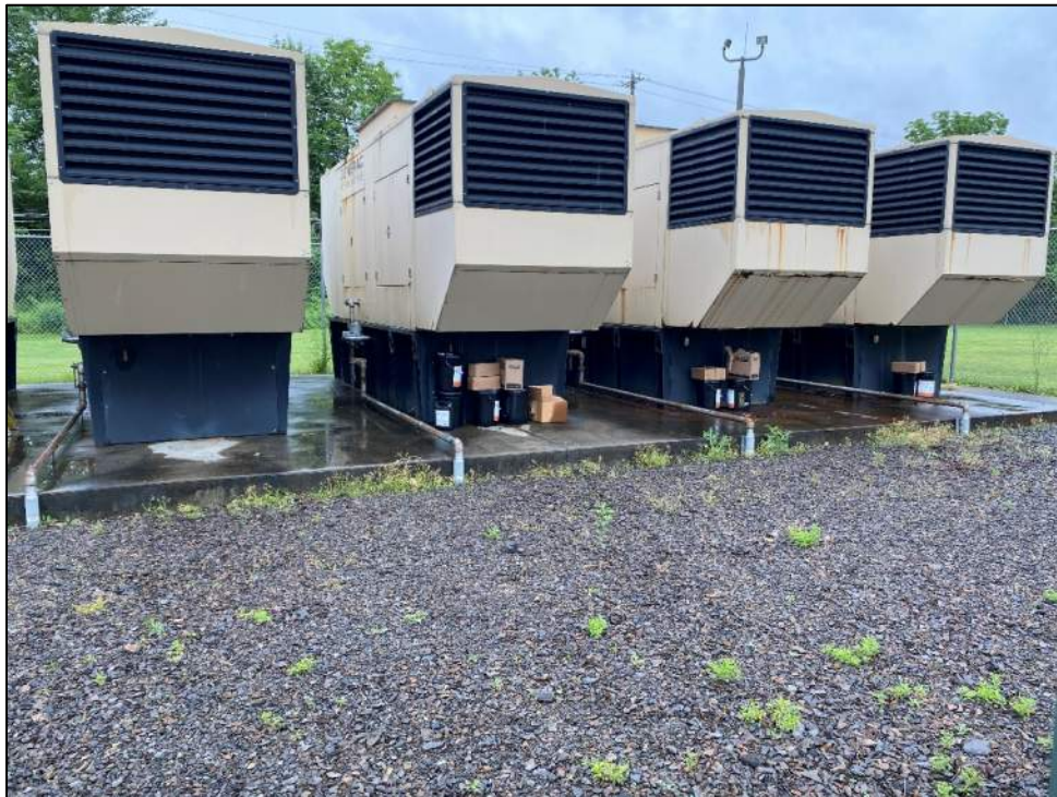
Photo 20: Generators in electrical substation area and eight 5-gallon buckets containing 15W-40 oil.
