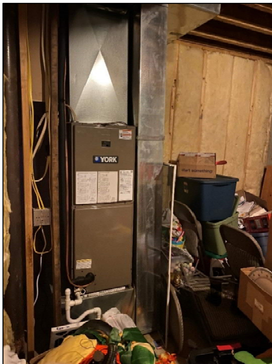
Photo 50: HVAC equipment in the basement of the residence.
