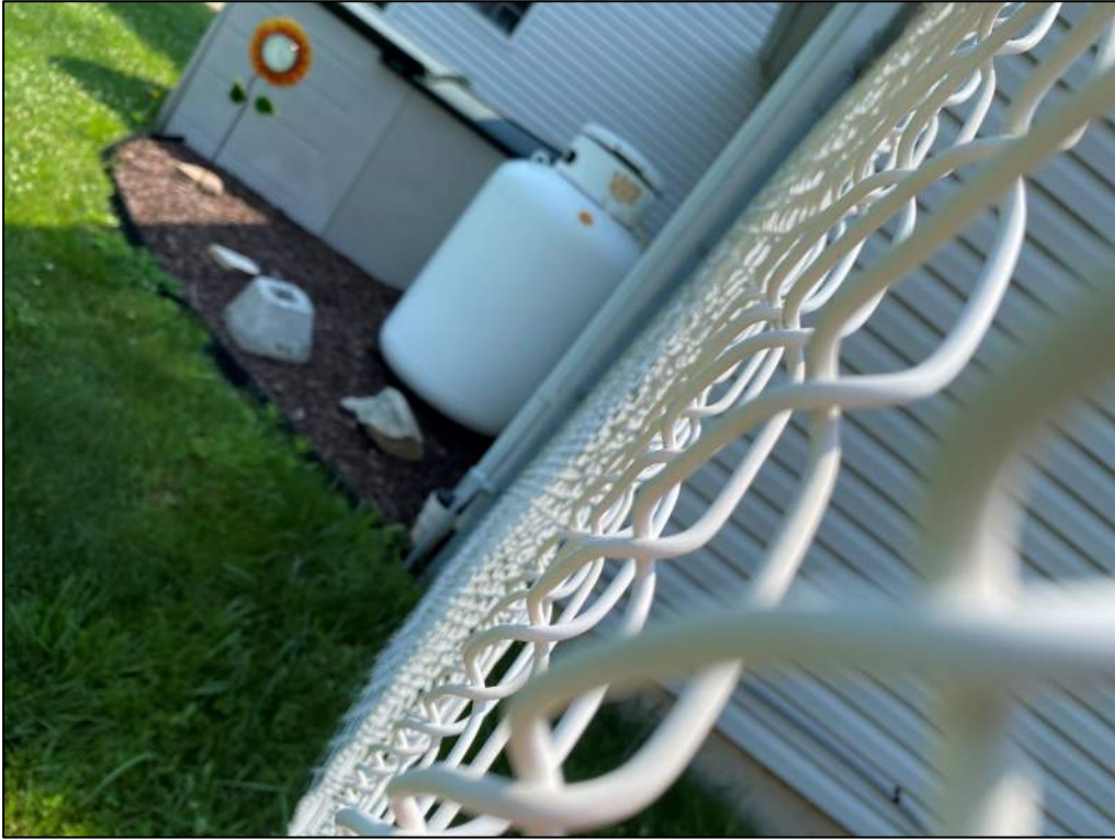
Photo 75: Propane tank in backyard of residence, likely used for indoor fireplace.
