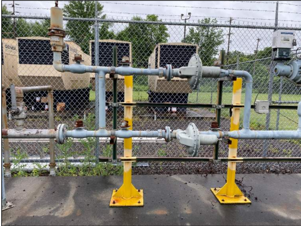
Photo 21: Gas regulator within fenced-in electrical substation area, facing west.
