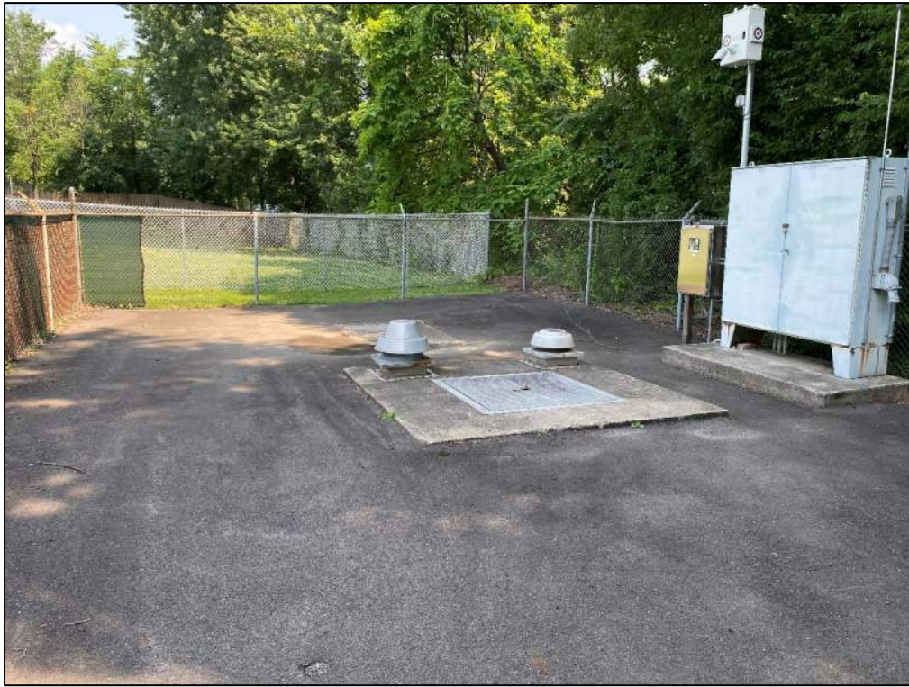
Photo 78: BCWSA substation at the east end of Central Avenue, facing northeast.
