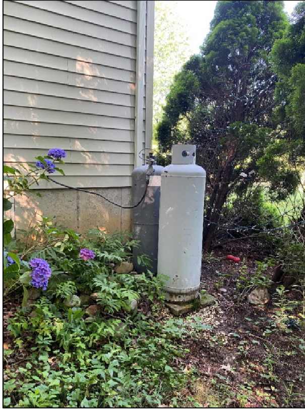
Photo 54: Propane tank on concrete pad for the inside fireplace located on the east side of the residence.
