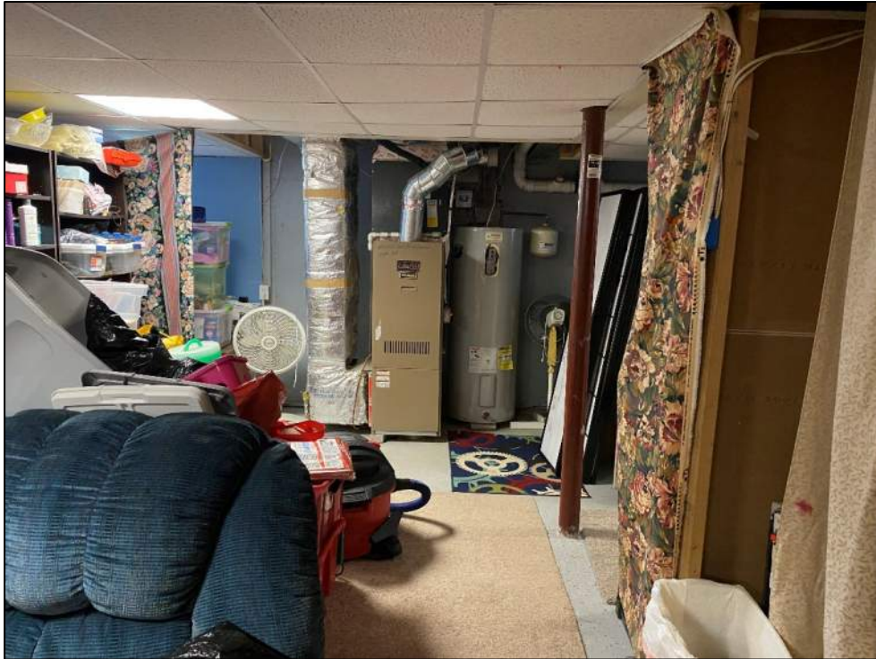
Photo 65: Water heater and furnace in the basement of the residence at 141 Central Avenue.
