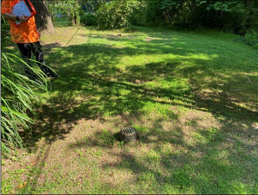
Photo 63: Vent pipe in front yard, likely associated with BCWSA sewer at end of Central Avenue.
