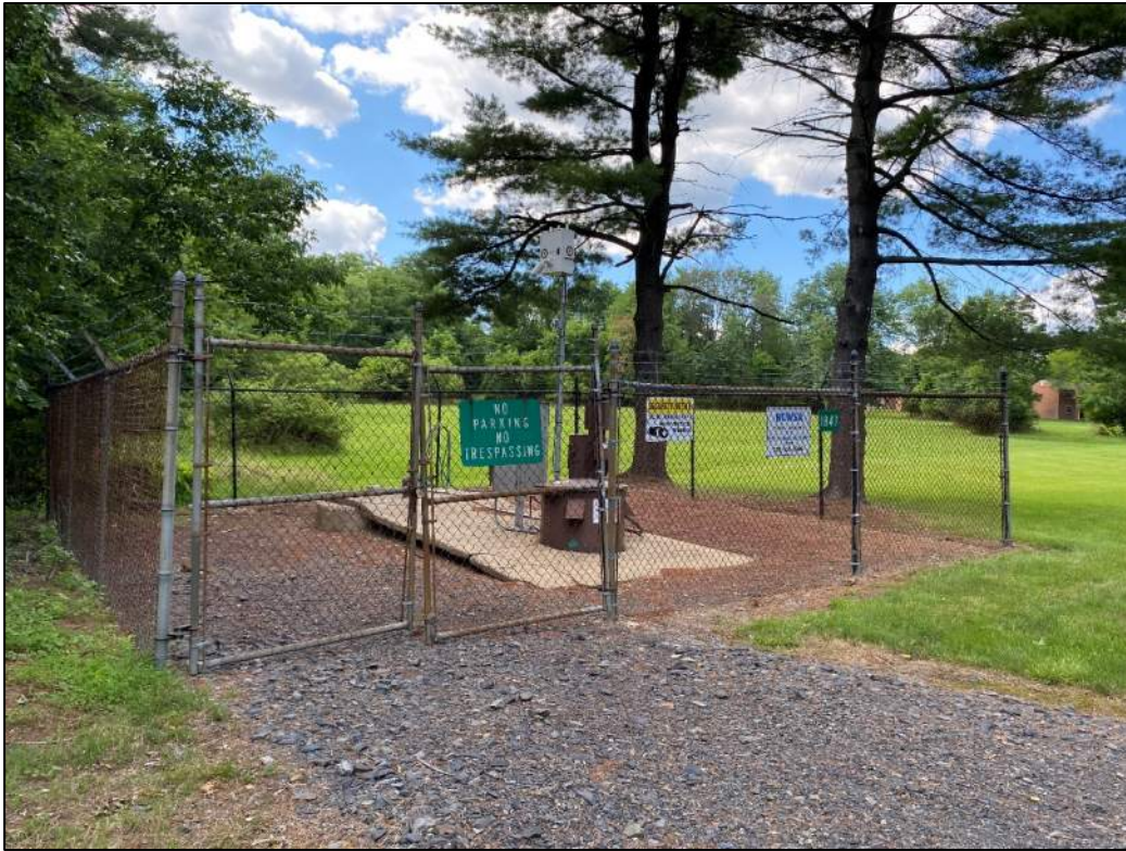
Photo 47: BCWSA substation along Old Lincoln Highway, facing northwest.
